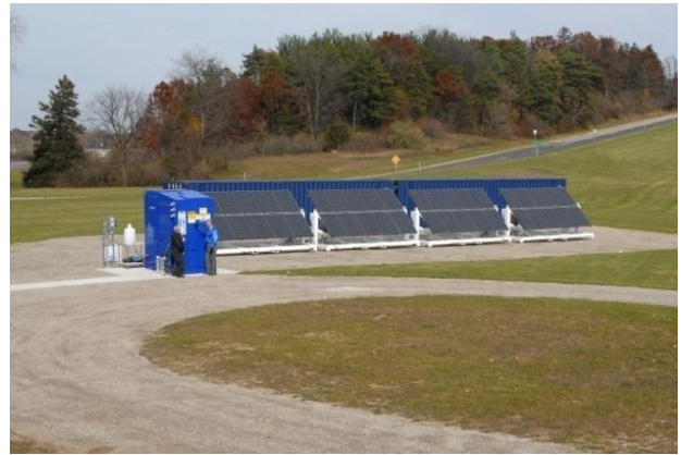
Figure 4. The combined PV-ESD (Electrolyzer, Storage, Dispensing) system, referred to as the GM Solar Hydrogen Fueller at the General Motors Proving Ground, Milford, MI.
